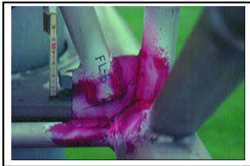
Figure 6:15-2: Gusset Plate With Fluorescent Penetrant
