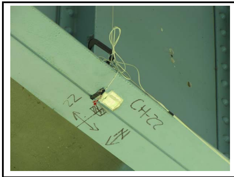
Figure 6-17-4: Strain Gauge on a Girder Flange
