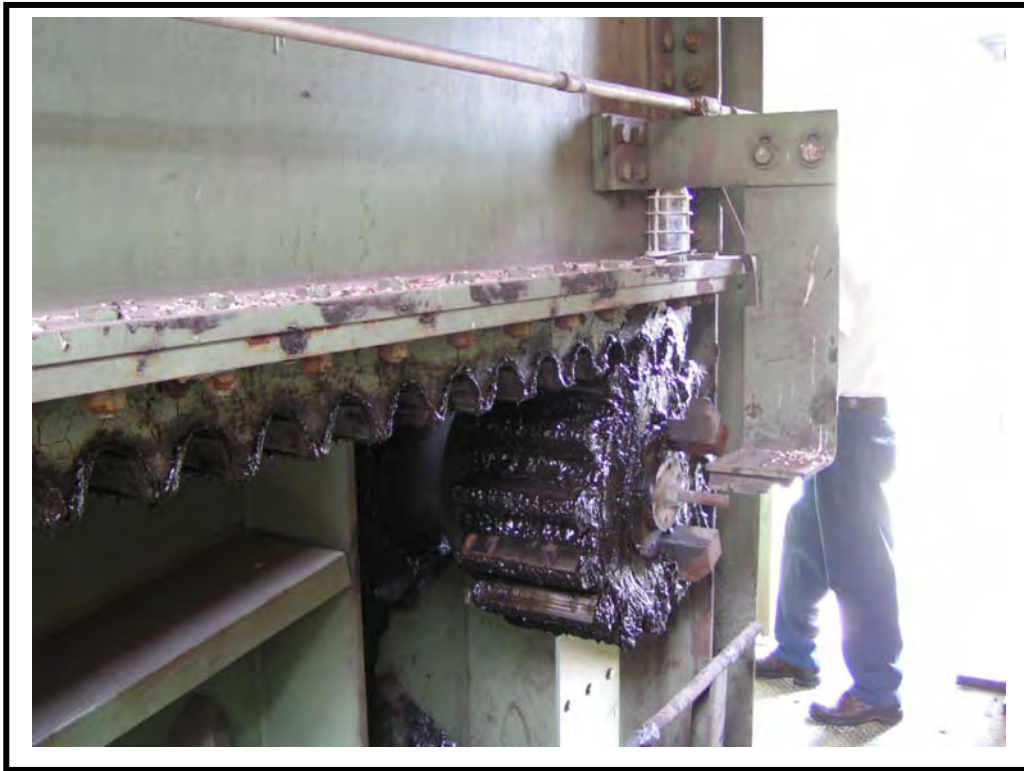
Figure 5:1-2: Rolling Lift Gears
