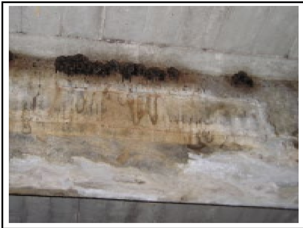
Figure 4:3-5: Bats Roosting Along Crack and Associated Staining
